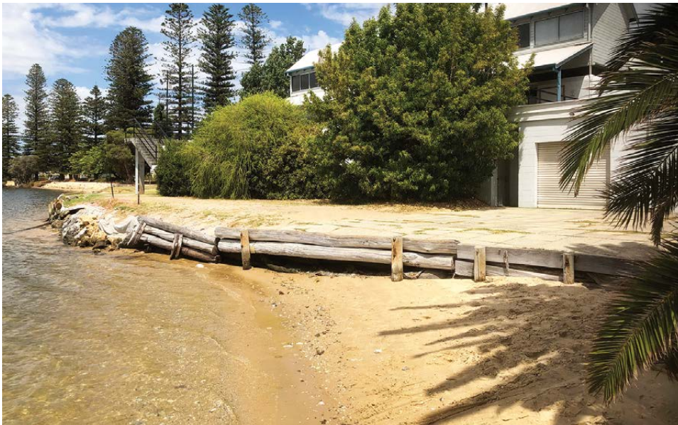
Over recent years, the shoreline at Apex Reserve had experienced erosion and the existing wall structures had severely deteriorated. Photo courtesy Advanteeing Civil Engineers
